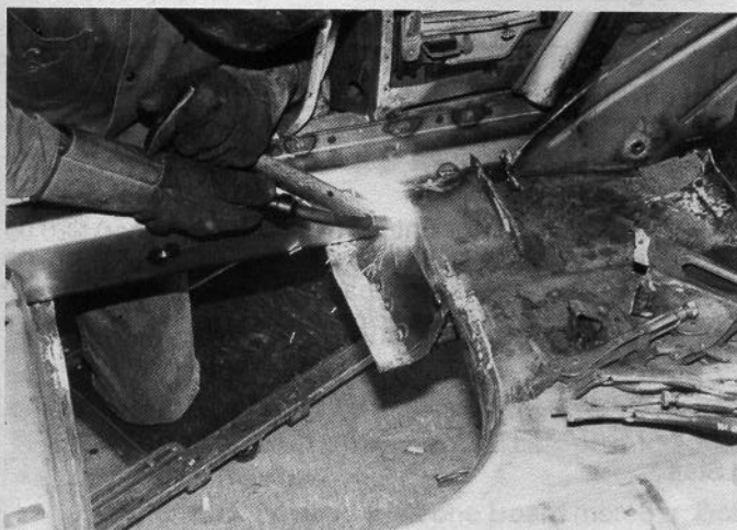
Skinner welds our plate into place. Once welded, he does the final penning into place. We're simply forming the plate to the torque box.
