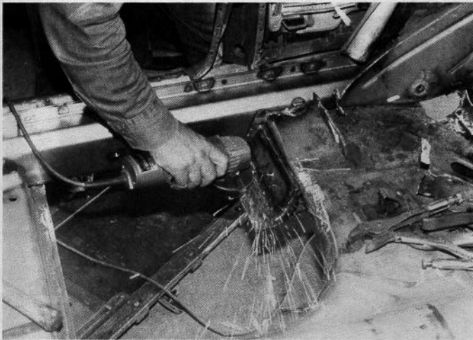
First, we clean up the mating surfaces with a grinder. Rusted surfaces will not weld. What's more, they will get worse. Clean it up first.
