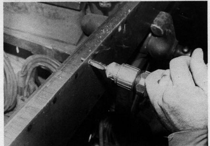
The new rocker boxes must be prepared for installation. Here, Skinner bores spot weld holes into the mating surfaces. Since we're not able to reproduce factory spot welds, we do the next best thing, we plug and fill.
