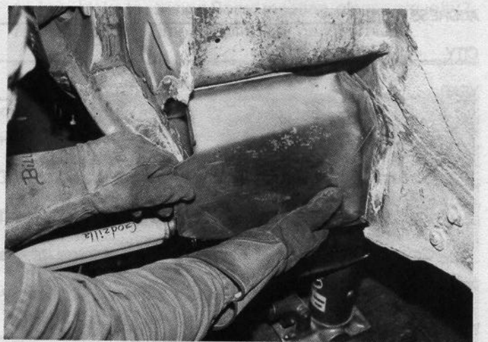
Next, Skinner fit checks the torque box. Notice the flange that is flush with the frame rail. The flange on the left (Skinner's left thumb) should be flush with the end of the outer and inner rocker boxes. Next month, more!
