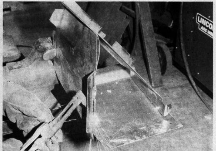
Some trimming of the front torque box is required in this case. As always, close attention must be paid to detail.
